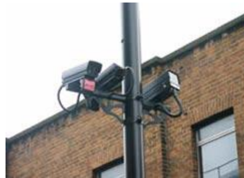
Pole Mounted Closed Circuit Television Camera
